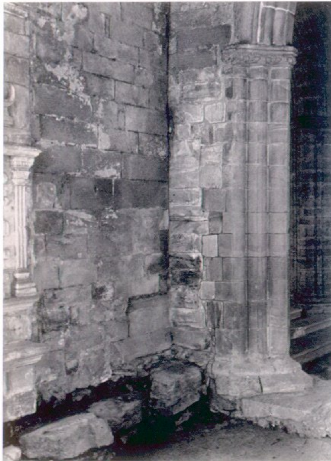
North transept: splicing of transept arch to older buttress Seton Collegiate Church.
