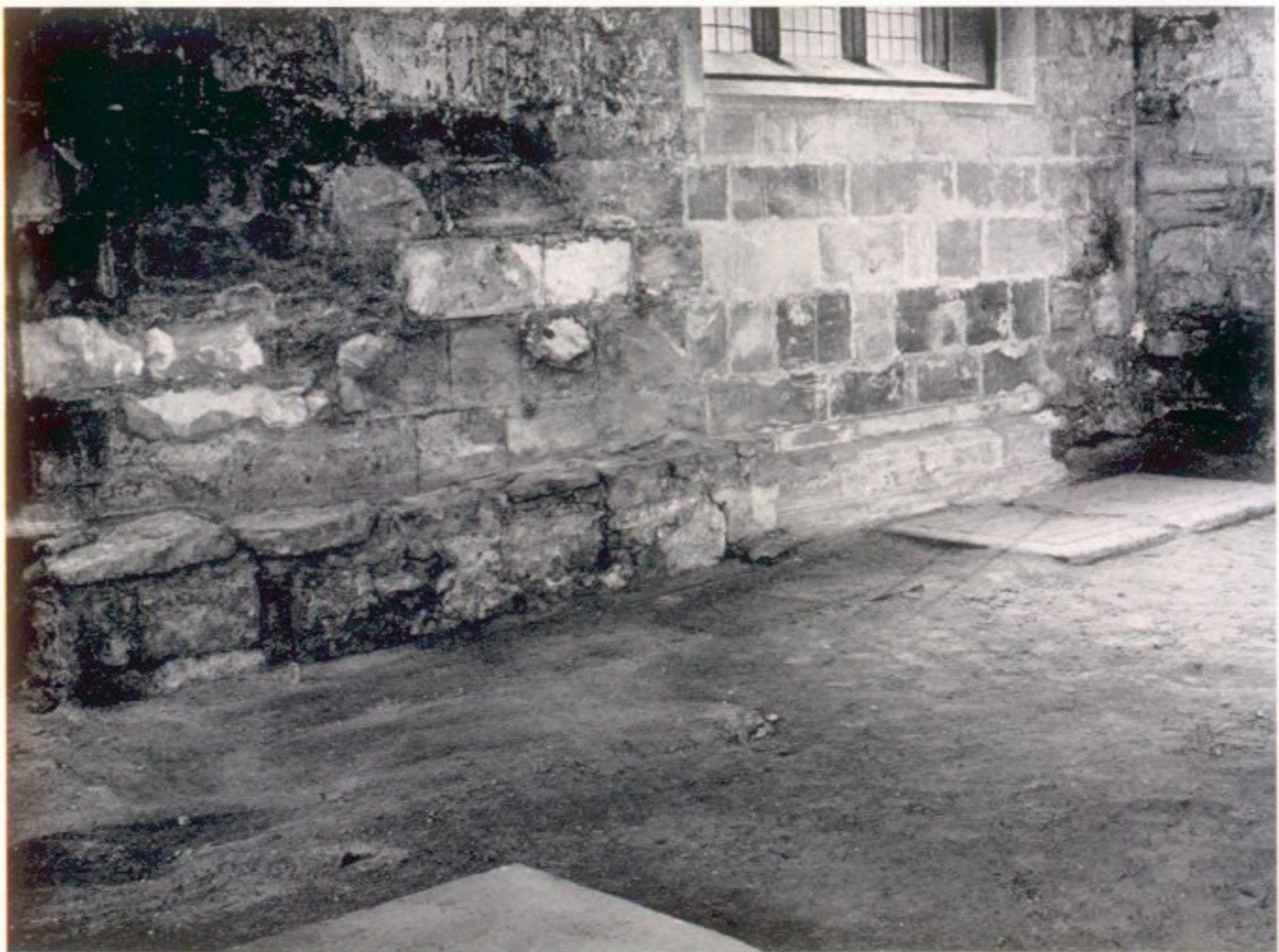
South-west corner of choir: showing lower floor, "benching," base of mural monument, rebuilt wall beneath window and gravestones.
